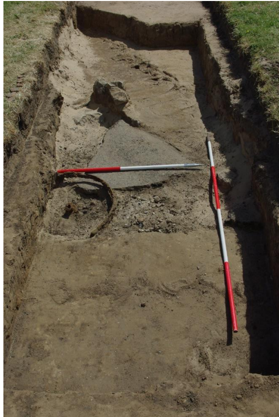
Figure 10: Trench 1 looking south with infilled gun pit in foreground, tarmac edging and the position of the sandbag revetment beyond. Note the front wheel of a motorcycle
